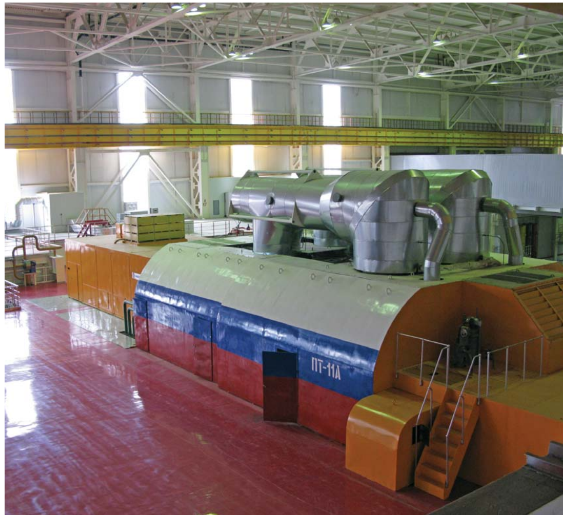
Asynchronized turbine generator T3FAU-160-2U3 with 160 MW capacity at unit 11 of CHP-21 by Mosenergo
