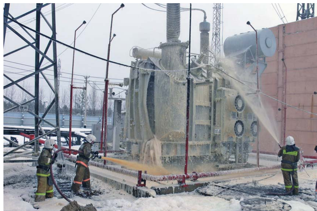
A North Siberian substation: transformer after explosion
