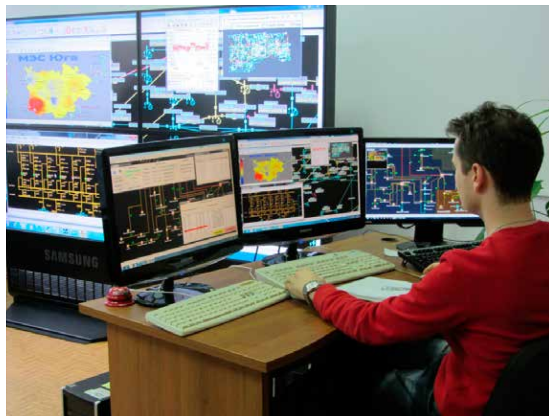
Digital substations are the forefront of technological advancements in the area of power grids
