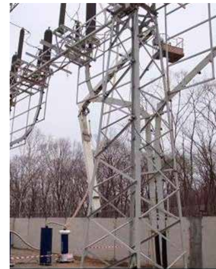
Fig. 4A. On-site testing of a 220kV 13.3km long XLPE cable circuit.
