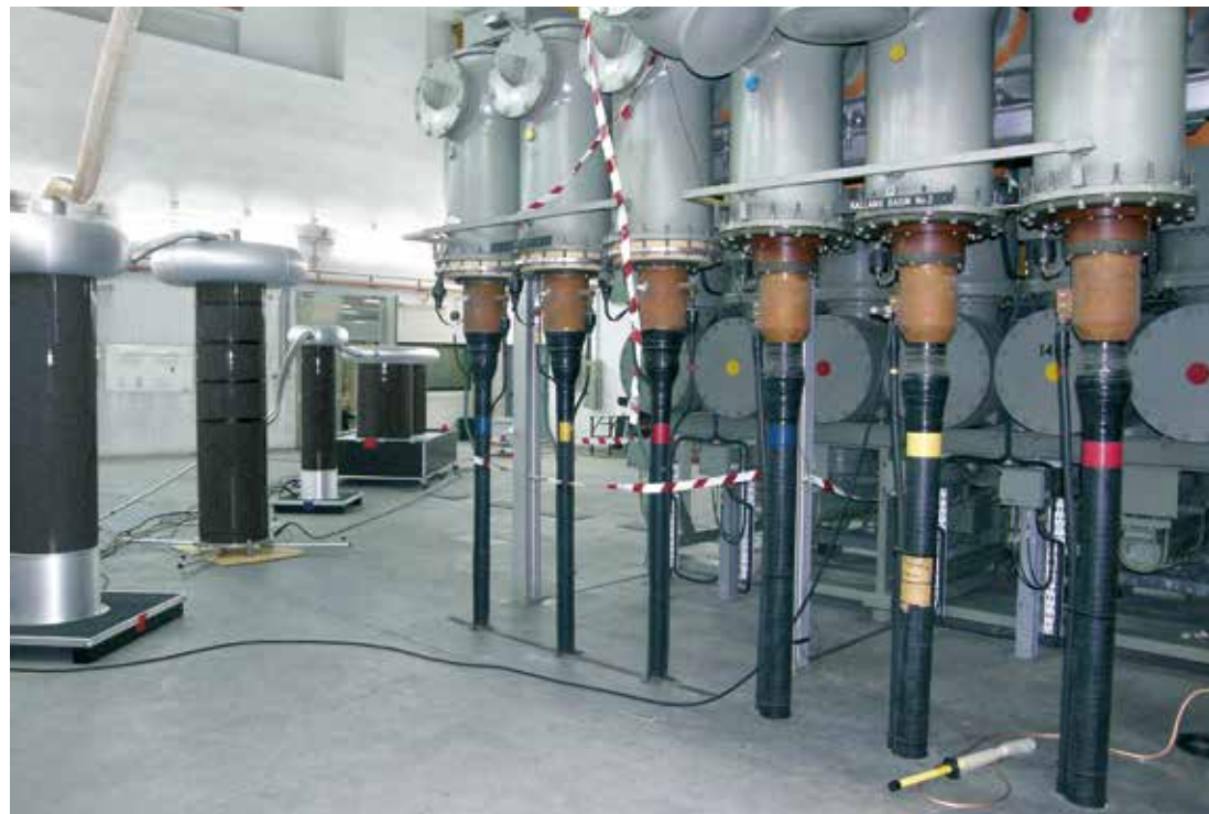
DAC HV40 system (for 500kV power cables) during testing of a high-voltage cable system in Singapore
