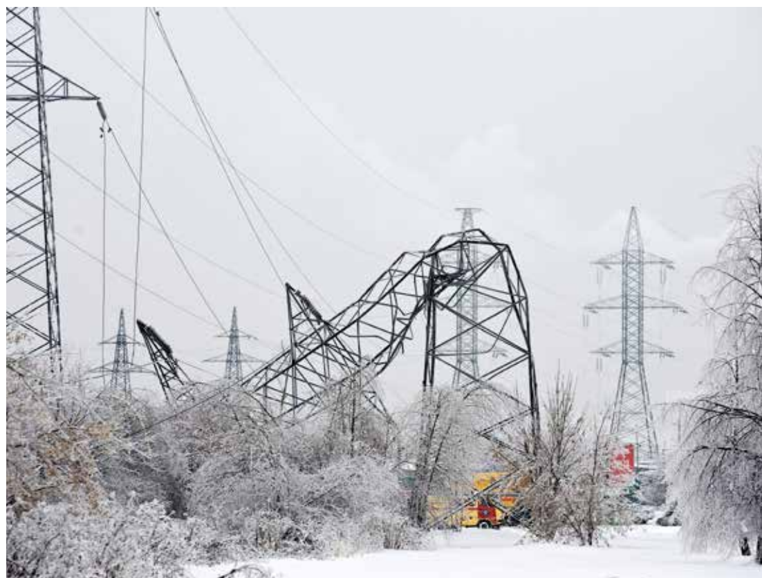
Transmission tower that had collapsed due to glaze ice near Vostryakovsky Lane, south of Moscow
